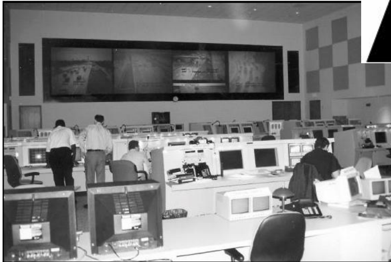
The Control Center of the TranStar Freeway Management System in Houston, TX.
